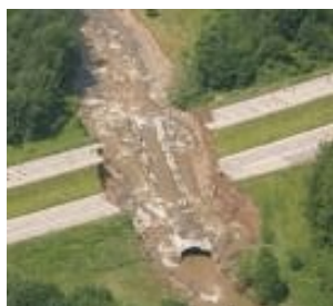
2006 Flood Damage Delaware County, NY
